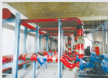
Fire Hydrant System
